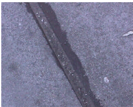
Above: handball court joint in need of repair.
