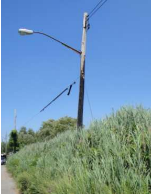
Figure 7: Fire scarred utility pole surrounded by Phragmites australis , Kissam Avenue
