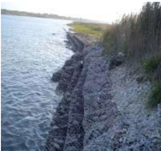
3. Toe scoured and "rolling," opposite ferry terminal.
