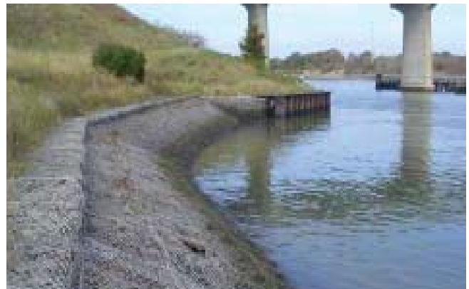
2. Sloped baskets with end wall return. Vandalism (hole) and algae buildup evident.
