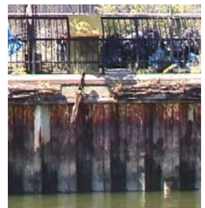
Rusting steel sheeting along Harlem River Park
