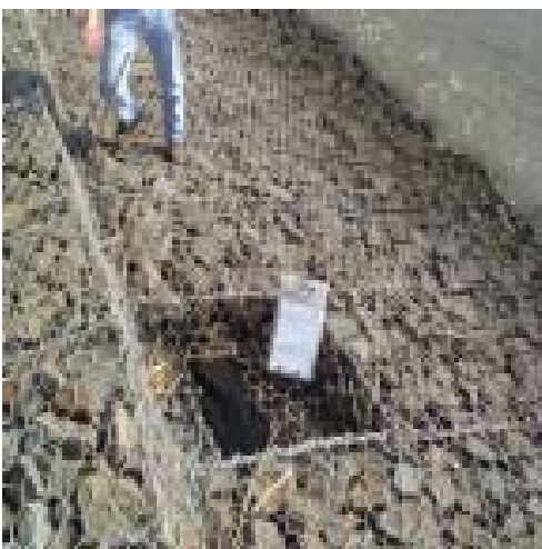
6. Vandalism: cut mesh and stones stolen.
