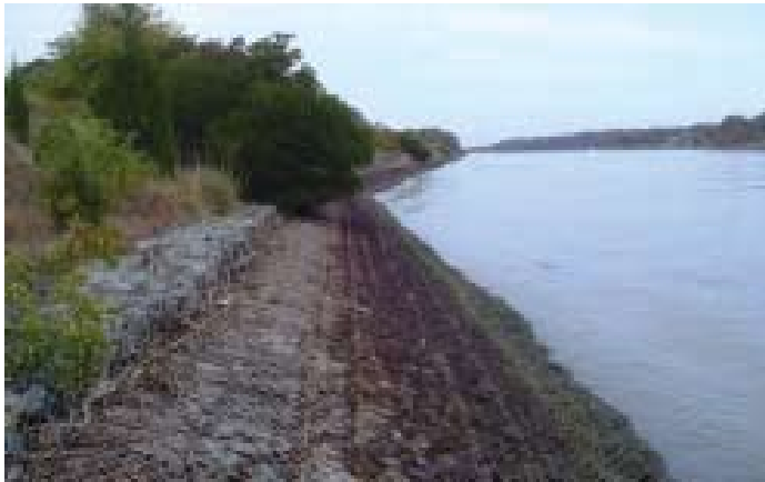
1. Rust in splash zone, double layer of mesh on top of sloped gabion blanket.
