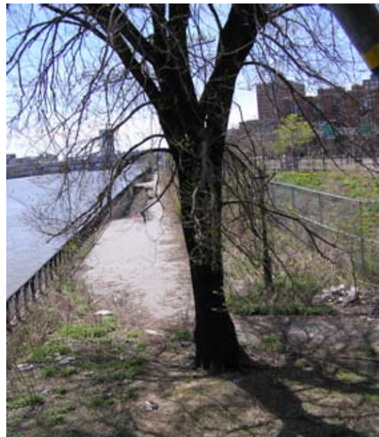
Preconstruction condition near 145th, showing collapsed esplanade.
